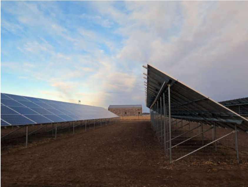
St. Cloud Utility's 220 kW Wastewater Solar Array St. Cloud, MN
